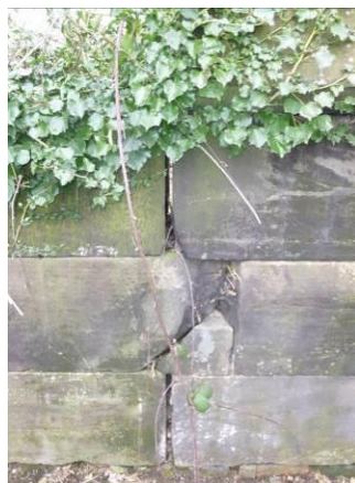
Crack and vegetation to bridge balustrade wall
